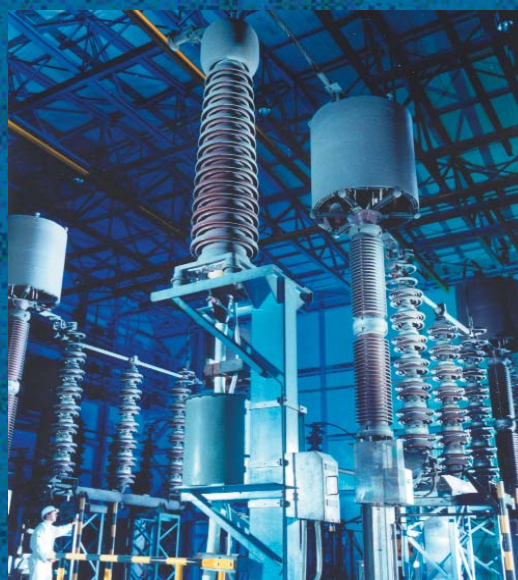
Peterhead Power Station
